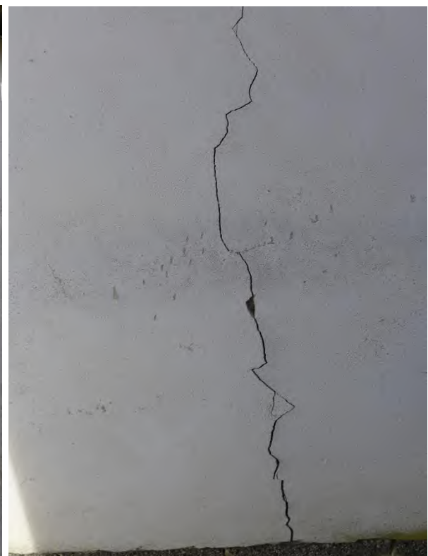
14 b Riss Garage
