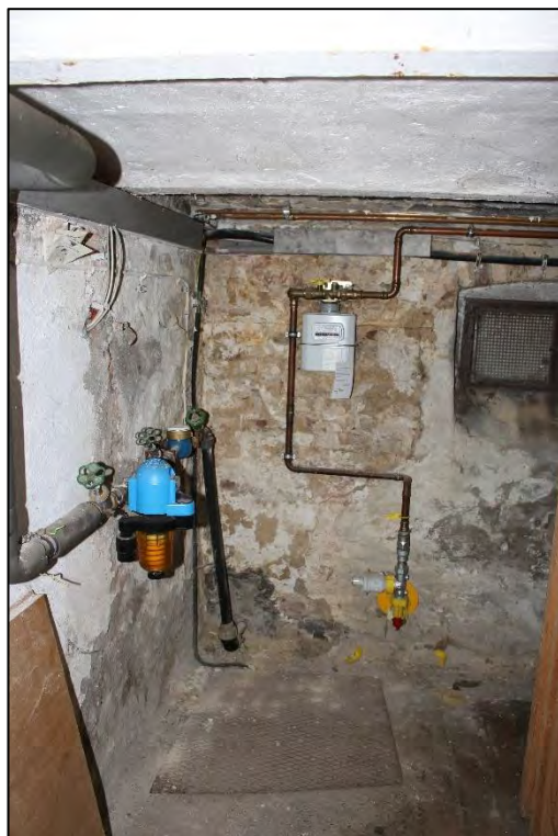
Foto Nr. 14: Kellergeschoss, Hausanschlüsse
